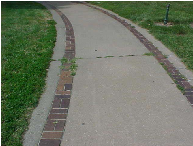
Weeds in sidewalk – Watson Park – Unsightly, and can damage sidewalk
