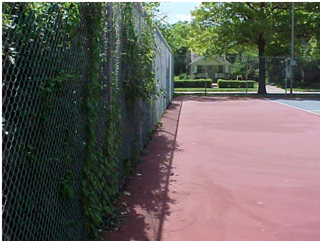
Weeds & vines in fence line of tennis courts – Veterans Park – weed control is necessary to preserve the fence structure
