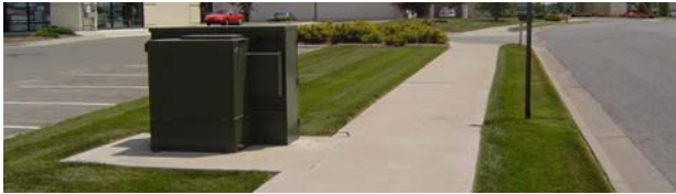
unacceptable location for mechanical equipment
