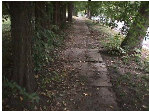
Debris on walk, some cracking
