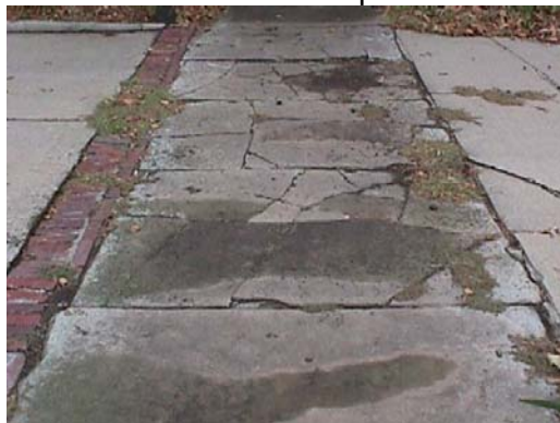
Slate walk, cracked
