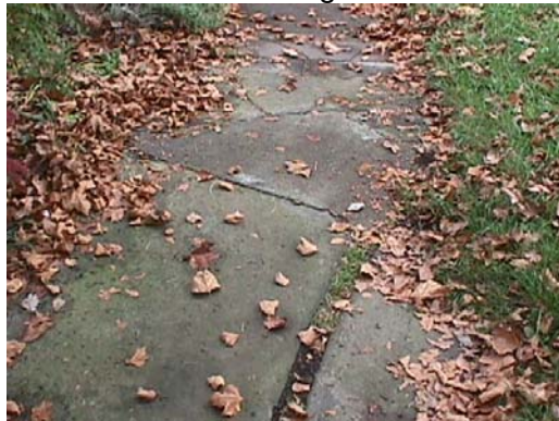
Slate walk with concrete patch
