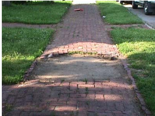
Bricks missing, trip hazards
