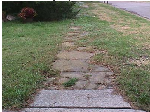
Slate broken and overgrown
