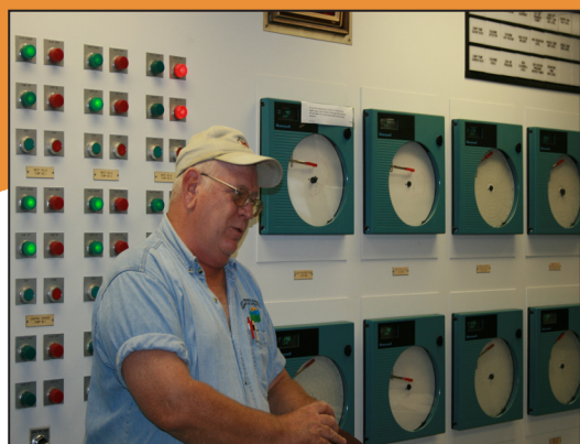
Twenty-four hour monitoring at the Clinton Water Plant keeps our drinking water safe.
