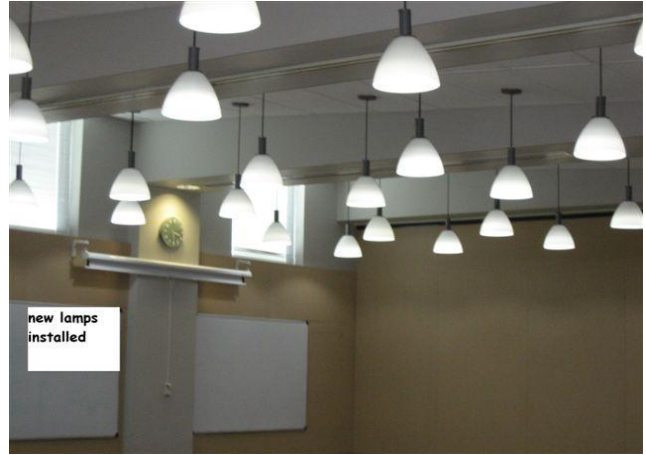
Health Building LED lighting
