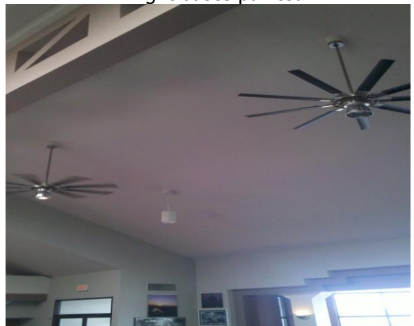
Ceiling fans Lawrence Airport Terminal
