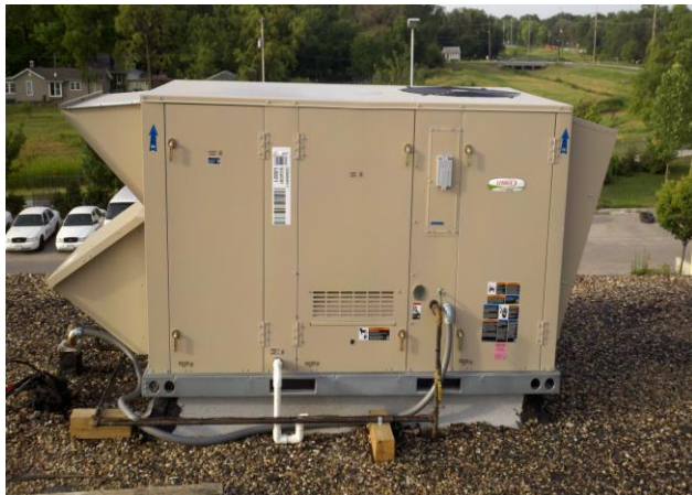
Central Maintenance Roof top HVAC
