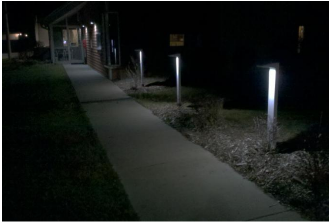
LED lighting Fire/Med #2
