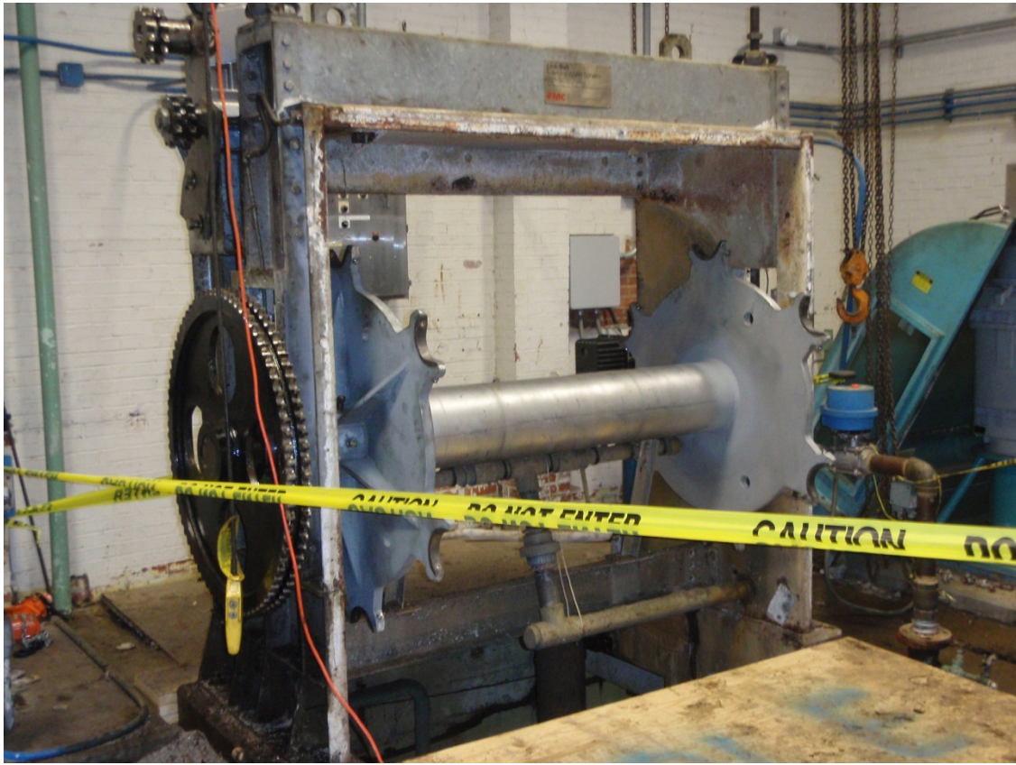
Traveling water screen head unit with new torque tube and chain sprockets installed.
