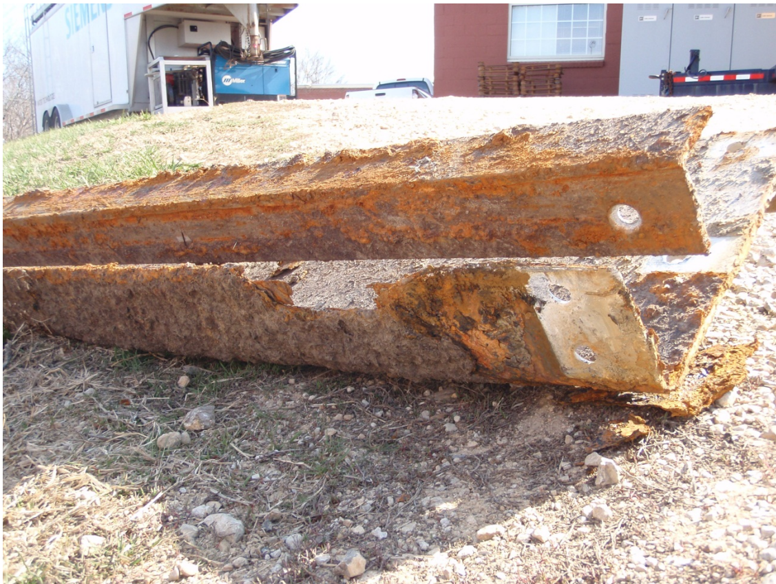
Corroded intermediate frame rail
