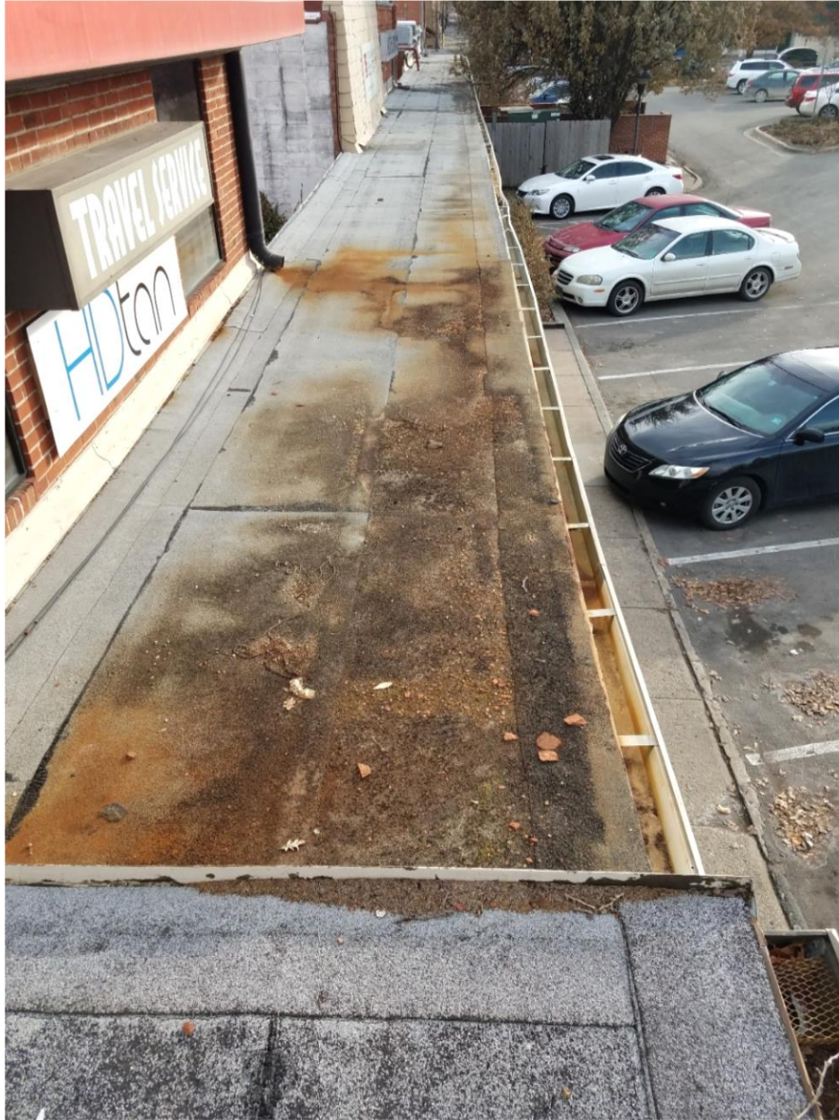
Typical roof section red stained areas indicate trapped water not shedding off into the gutters
