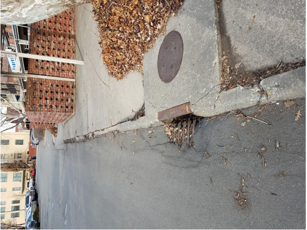
Storm water inlet with concrete settling and trip hazards
