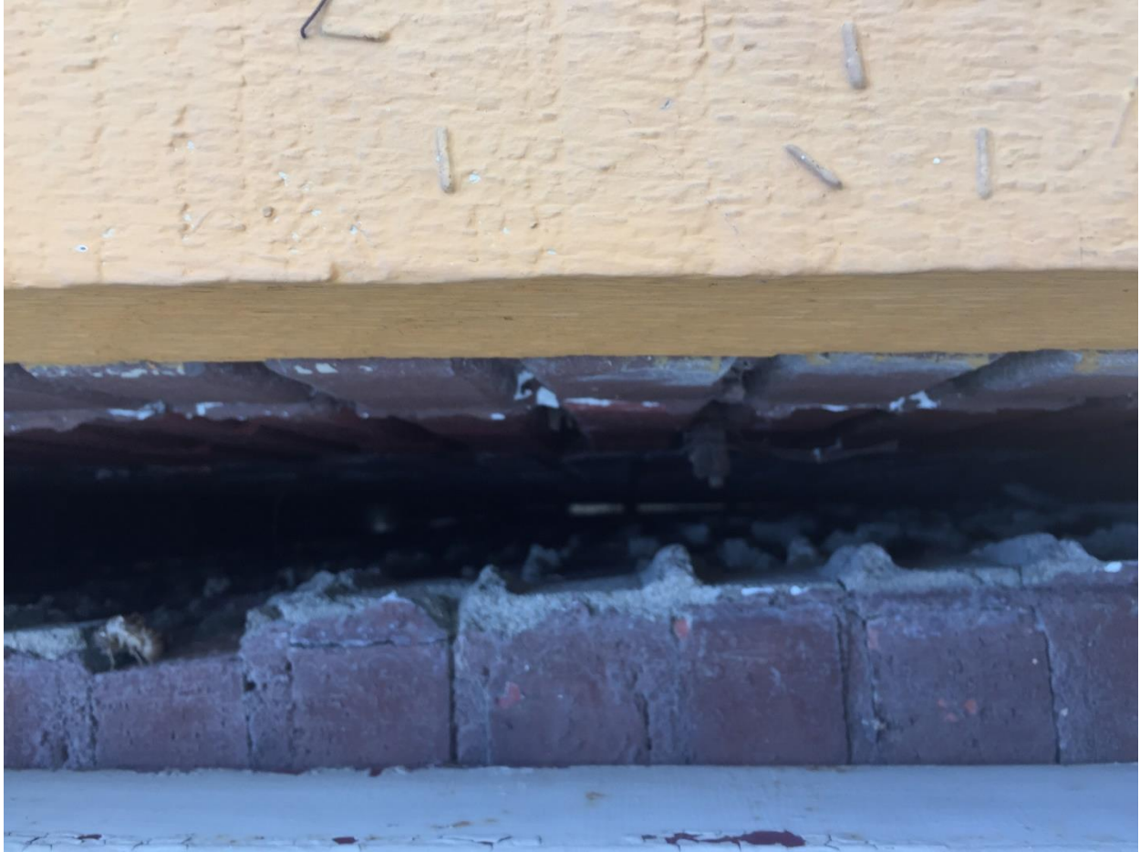
Brick Façade section separating from original structure. Structural steel members of the Canopy are the only thing keeping it from falling down (Could not rotate picture, this is vertical wall section)
