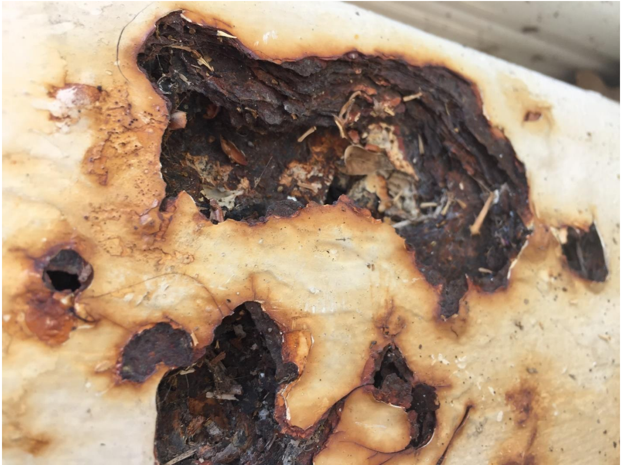
Structural steel column rusted through
