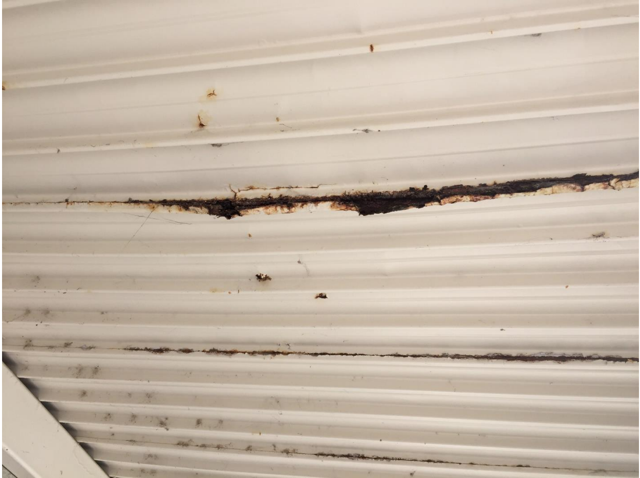
Metal roof decking rusted through and leaking water
