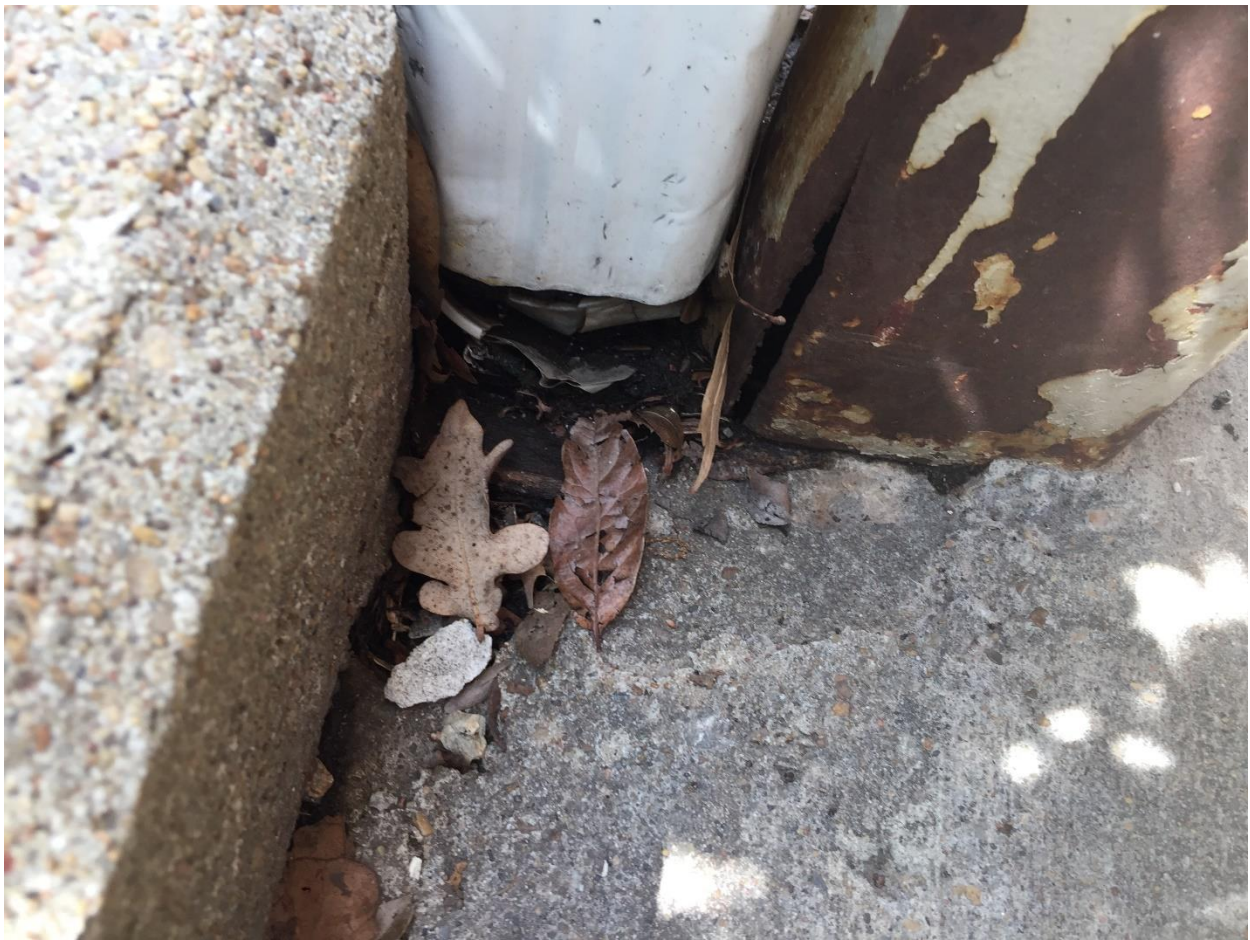
Structural steel column and storm water down spout. Structural steel cracked and rusted from freeze thaw water infiltration. Gutter and storm water inlet plugged.
