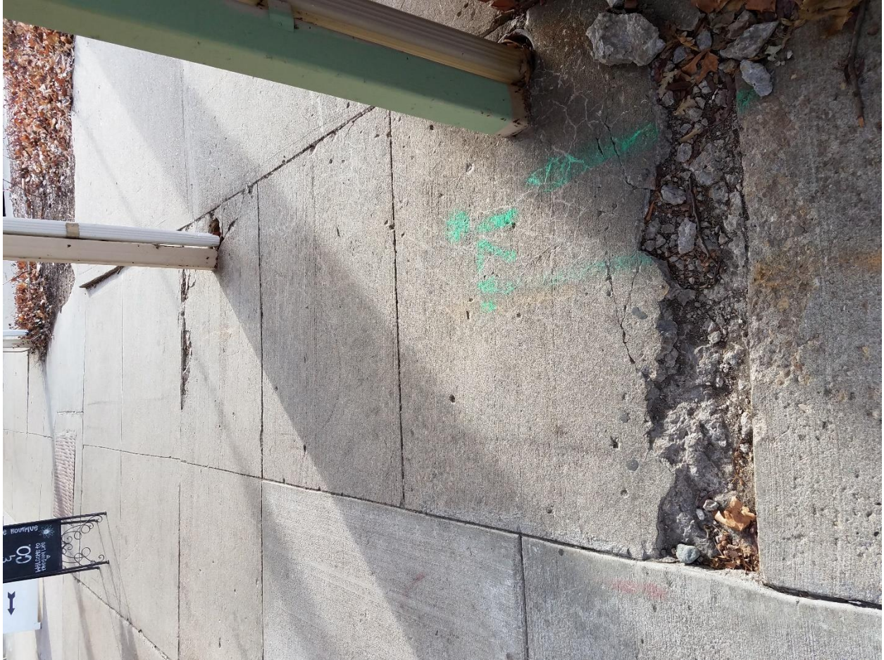
Typical concrete trip hazard and replacement issues (could not rotate picture, This is sidewalk under the canopy structure)
