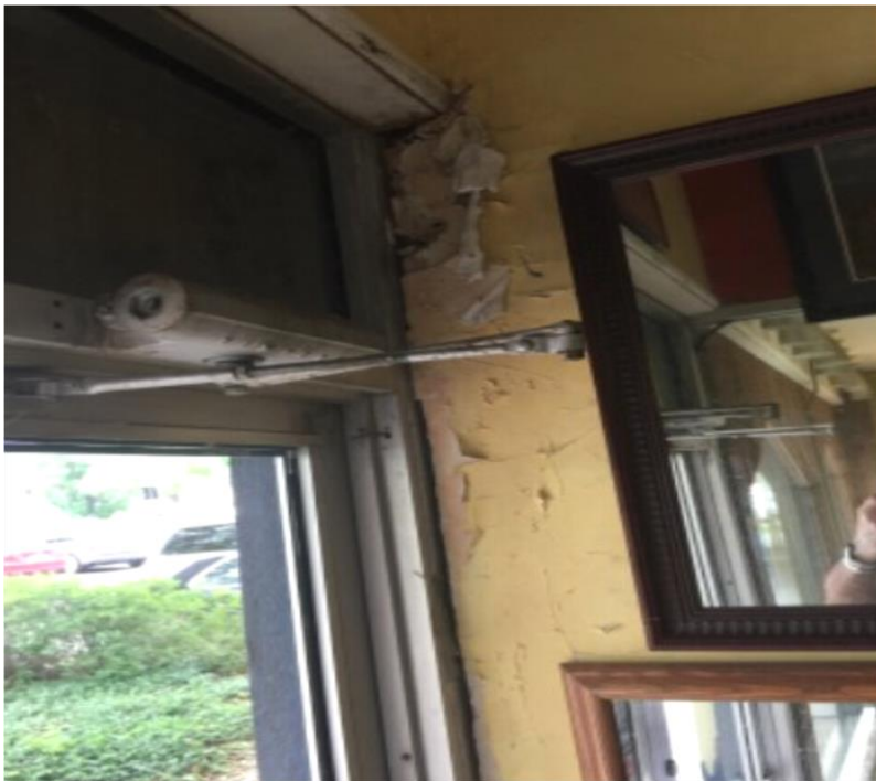
Water damage to the interior of buildings due to canopy water runoff
