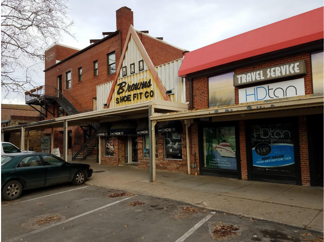
Typical Canopy sections. Gutter and Downspouts in disrepair
