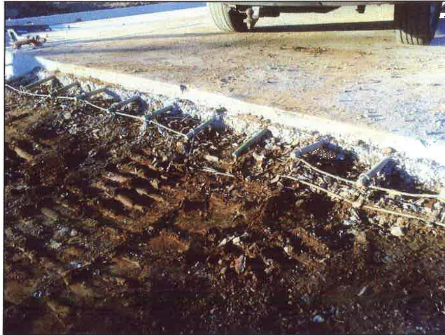
Bent dowel bars.
